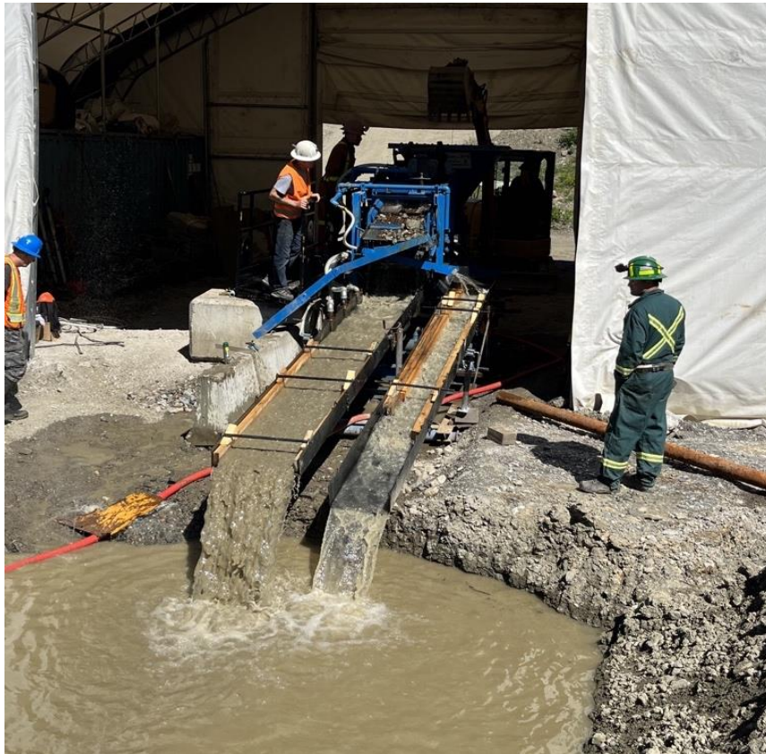
Backend of Wash Plant – Boil Boxes
